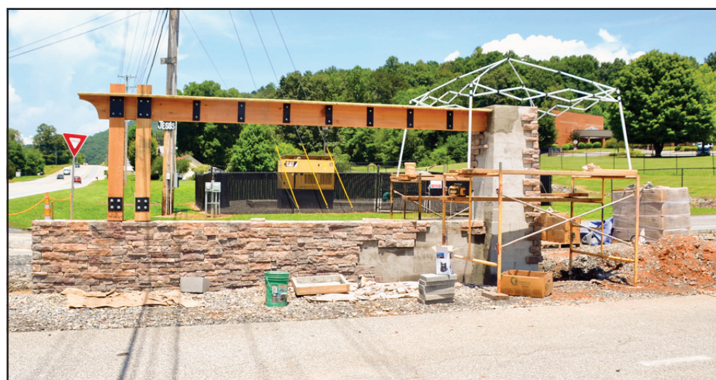
The new sign at the entrance to Towns County Schools is well on its way to completion, replacing the 40-year-old sign that had been around since the campus was built. Photo by Lowell Nicholson
